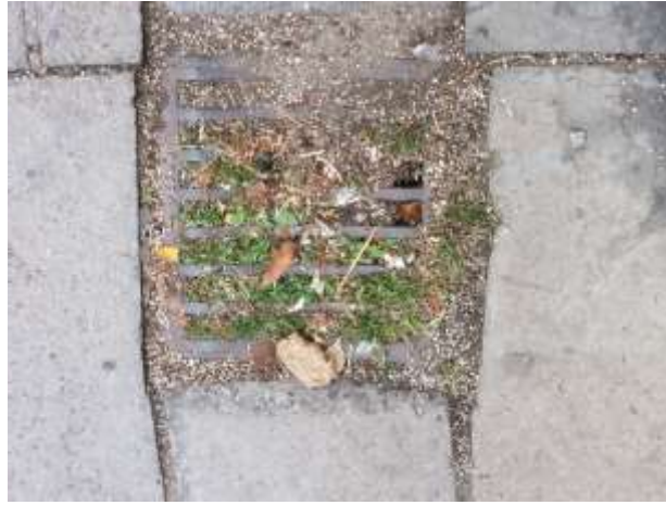
Blocked drain High Street
